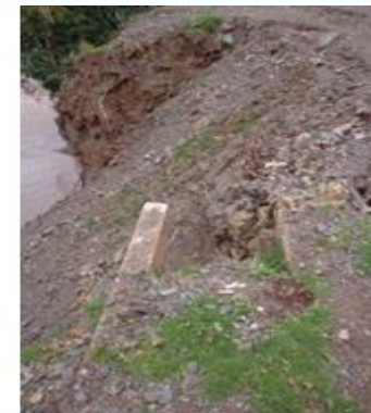
Canal principal revestido Accarani colapsado (PER Plan MERISS, 2013a).
